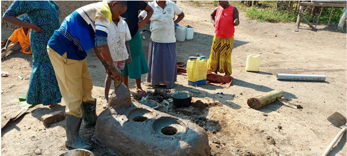
Photo 7: A field supervisor demonstrating stove construction techniques to the community members in Njagaazi © by Jjemba (July, 2024)
