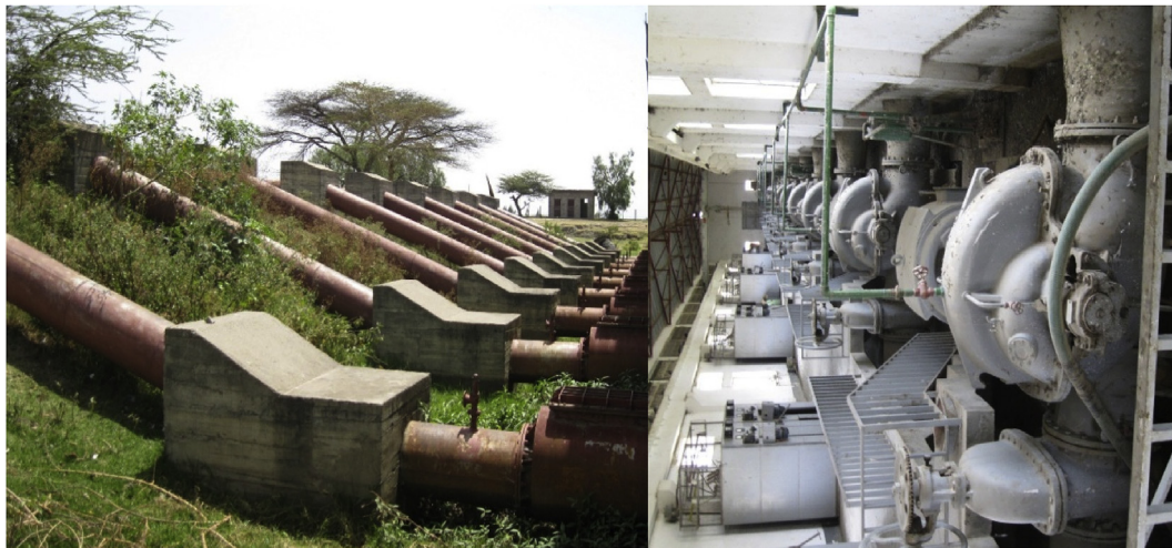
Fig. 11. Electric pumps being used for irrigation at Meki.
