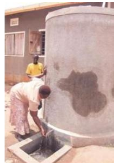
Right: Headmistress of Nakasongola SSS tapping water from the erected tank- proof that rain water harvesting is in progress.
