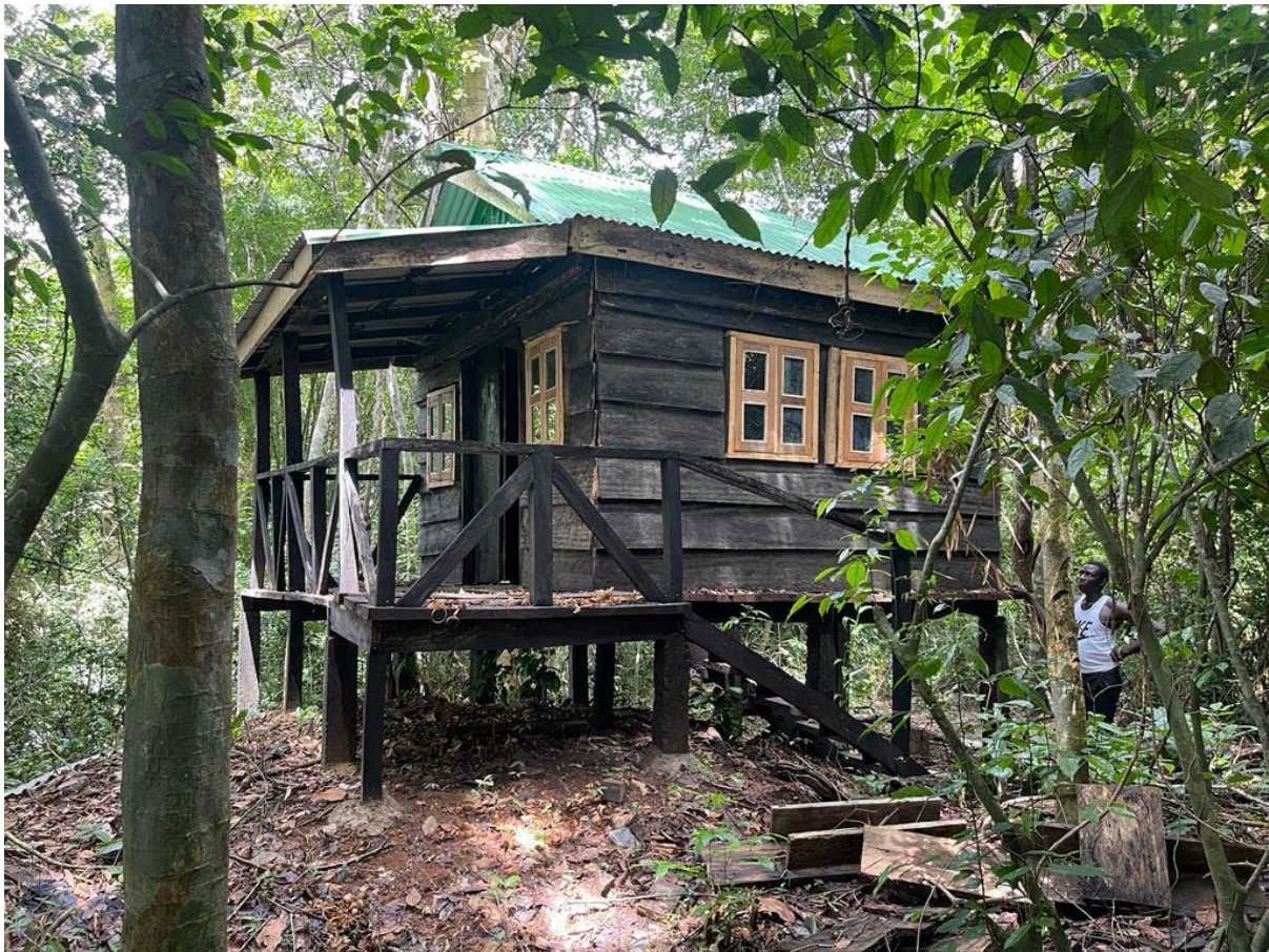
Newly constructed ecolodge at Jaibui Island by the Tacugama Chimpanzee Sanctuary. © Ambrose Bockarie Kanneh.
