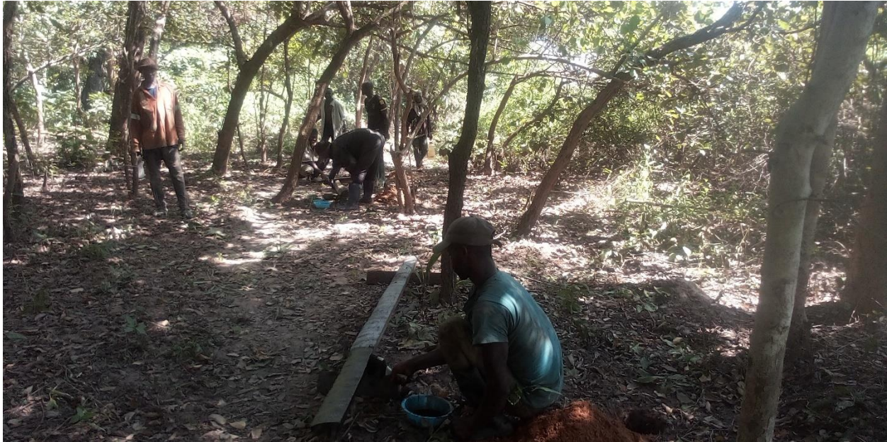
Plate 2. Digging of holes and treatment of wooden posts against insects using used engine oil. Credit: Ishmael Hashmiu
