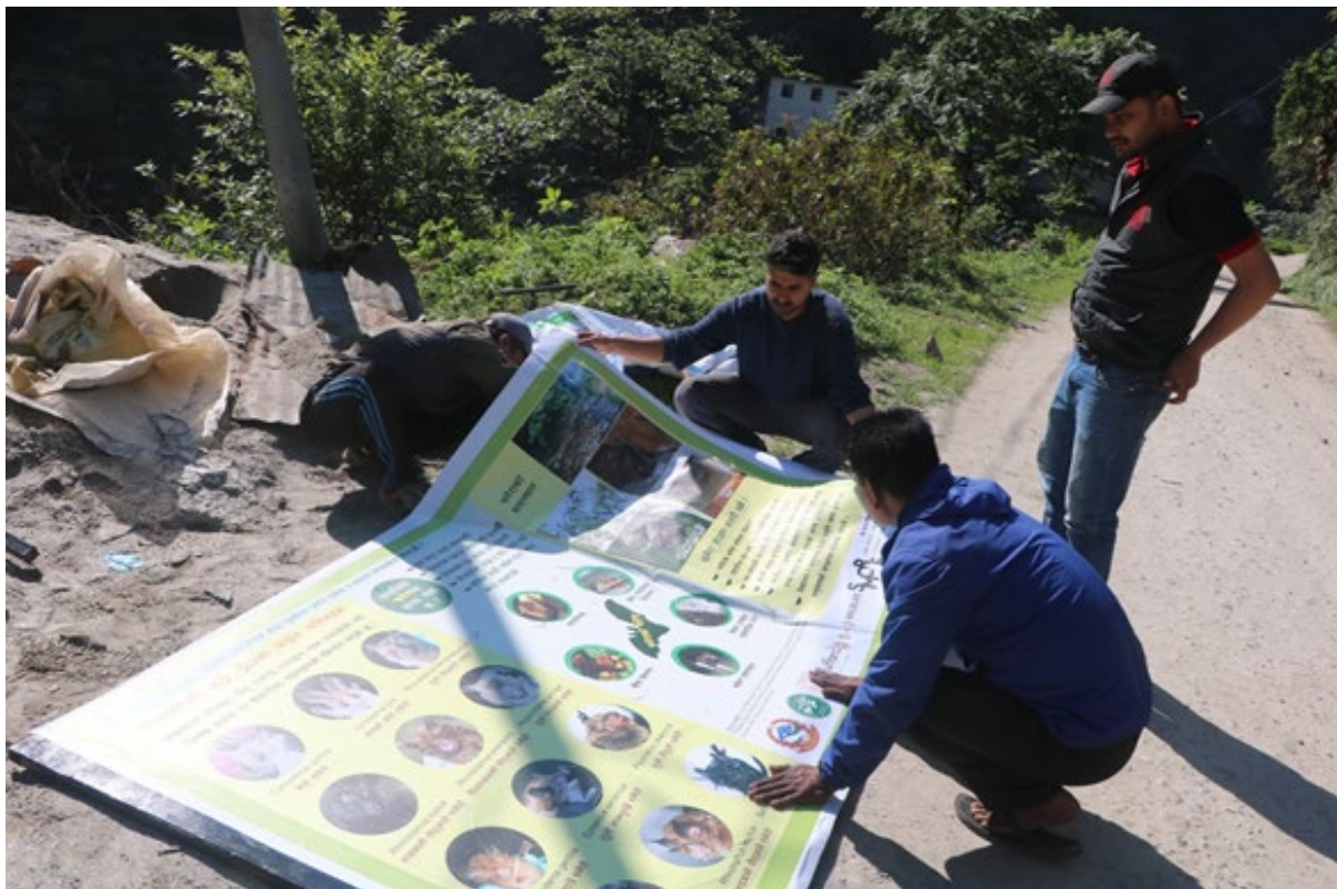
Figure 16: Pasting UV print flex on the metal board frame before installation with the help of locals.
