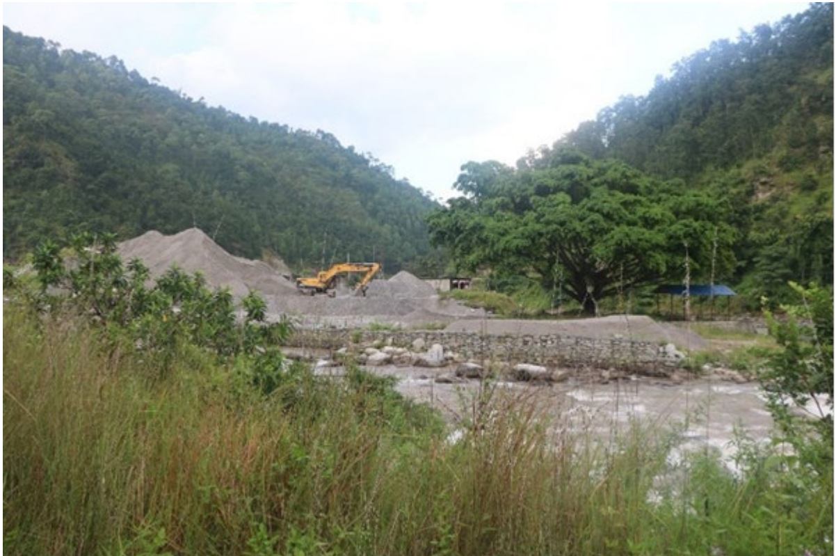
Figure 19: Sand and gravel extraction being done in Tamakoshi River near Tamakoshi Bajar, Dolakha district.
