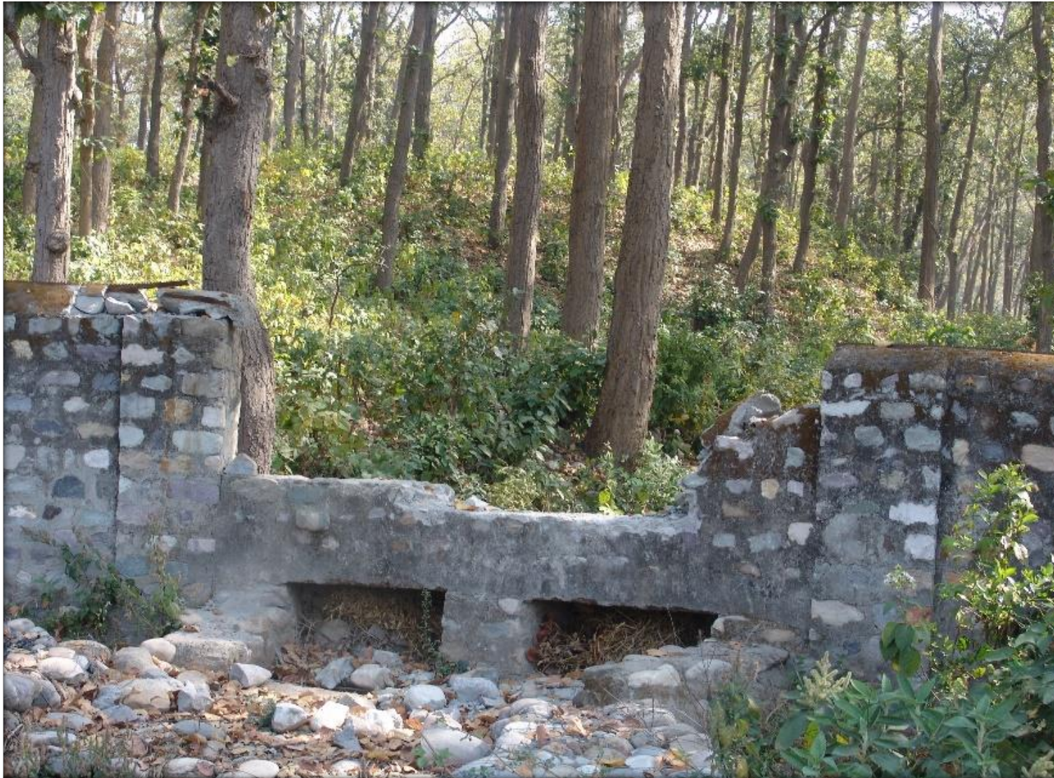
Appendix 4. Boundary wall damaged by elephants in the Ramnagar forest division.
