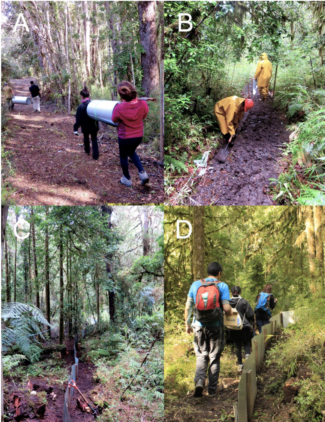
Figure 1 Installation of the exclusionary fences, a mitigation action against chytridiomycosis in Darwin's frog populations. In A) fieldworkers move the aluminium sheets used to build the enclosures. In B) a fieldworker is digging the ditch required for the fence during a day of harsh weather. Fences that have been successfully installed are shown in C and D.
