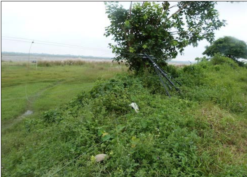
Figure 2: Grasses and climbers covering solar-powered fence in Bahundangi VDC
