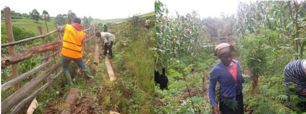
Left: Construction of the seed bank fence. Right: Integrating agroforestry tree seeds into crop farms
