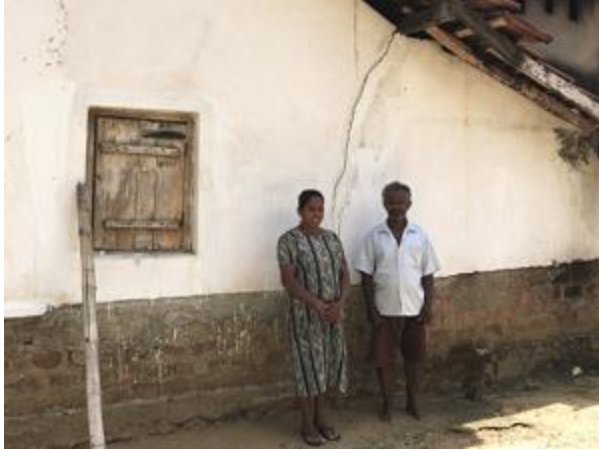
Figure 2 - Mr and Mrs A.G. Ariyadasa standing outside their home. The crack in the wall was caused by elephants trying to break in to steal sacks of rice stored inside, Mrs Ariyadasa was inside at the time this incident occurred.
