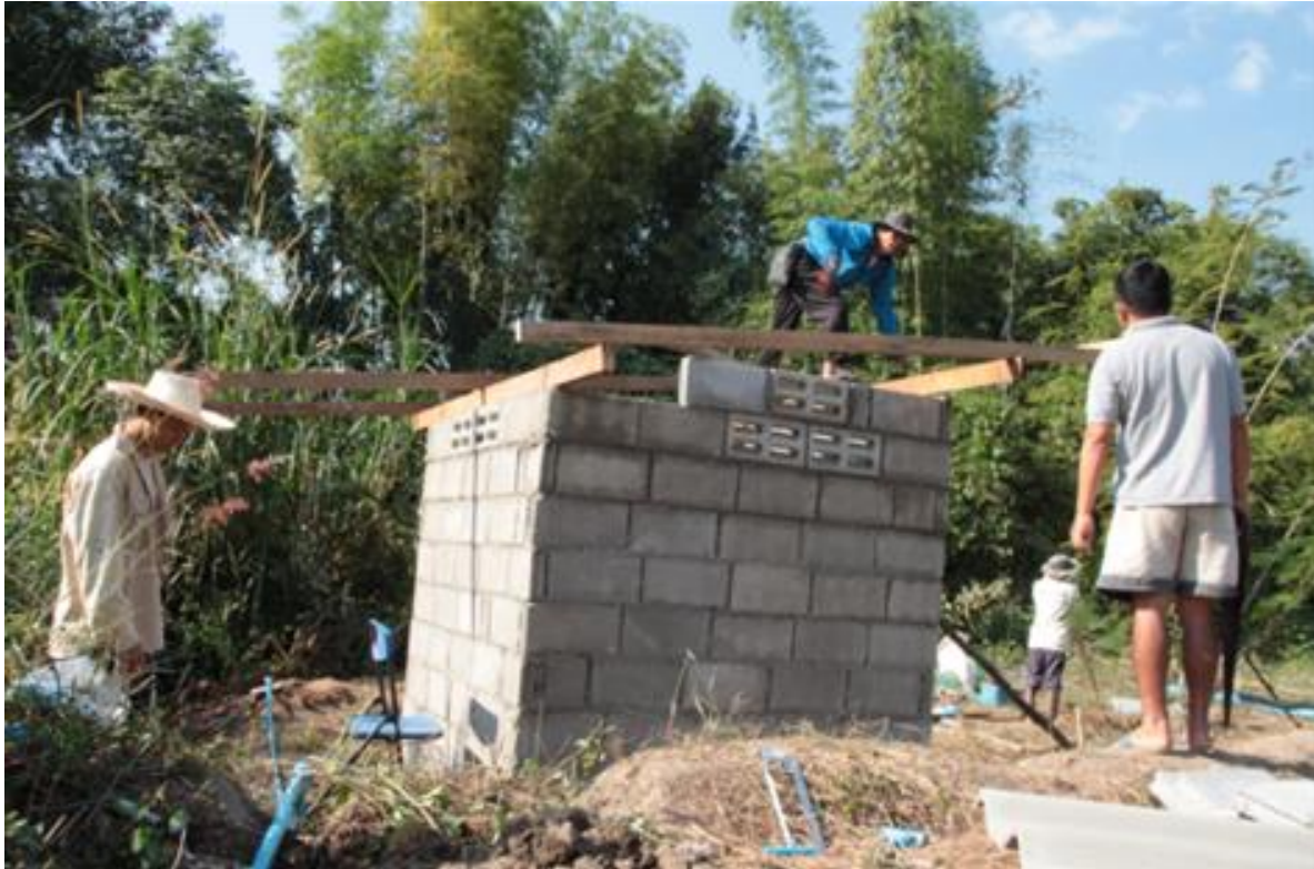
Building toilet and water system
