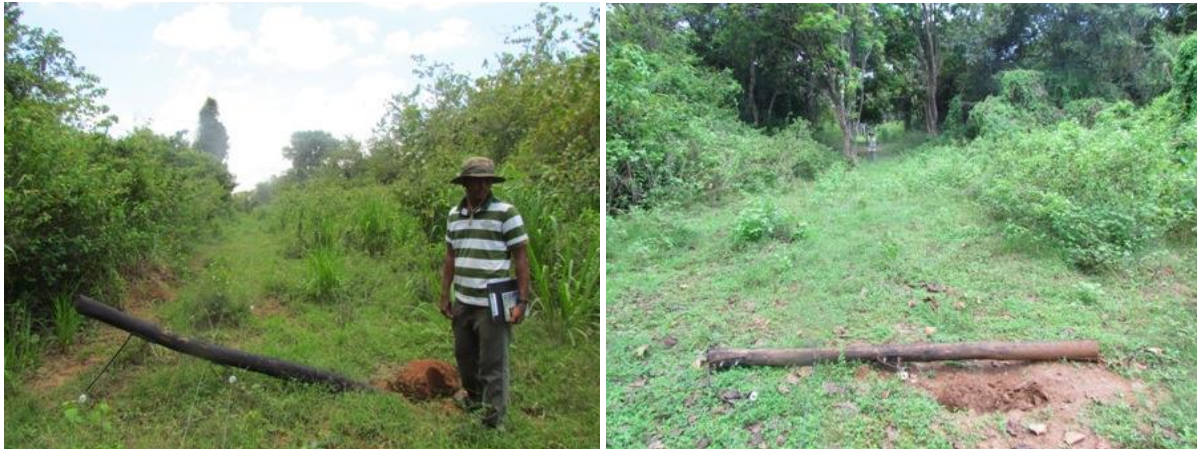
Plate 3: Fallen posts of the park electric fence.
