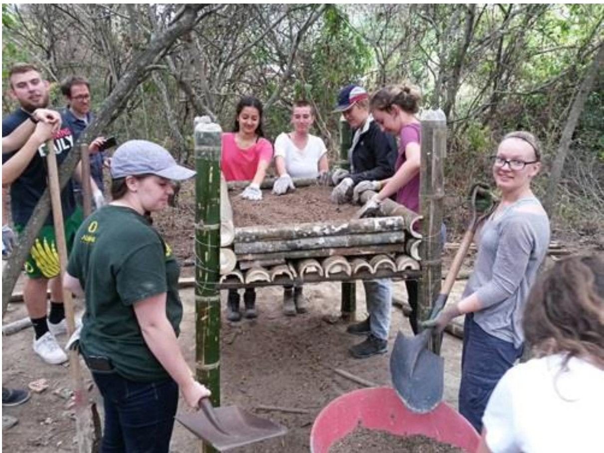
Students from a University of Oregon study abroad program construct and plant an elevated seedbed at the Planet Drum greenhouse.
