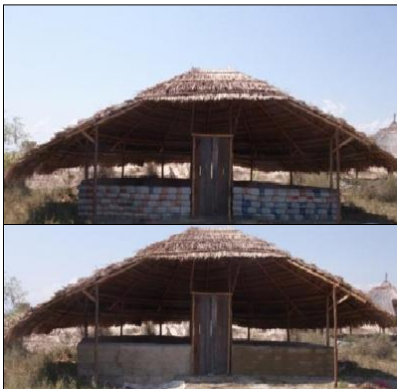
FIGURE 4: THE EDUCATION CENTRE DURING ITS CONSTRUCTION PHASE, AWAITING MATERIALS FOR THE FINAL SECOND STAGE OF THE WALL BEFORE IT IS COMPLETE. THE TOP IMAGE SHOWS THE MAIN CONSTRUCTION WORK COMPLETE WITH DOORS, THE LOWER IMAGE IS AFTER RENDER HAS BEEN APPLIED TO THE BAGS THAT WERE USED IN THE BUILDING.
